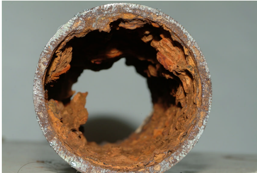
Figure 3. Large MIC Nodules in a Wet Fire Sprinkler System
