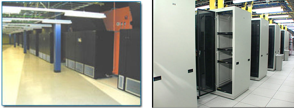
Figure 6. Leaks above Data Centers like these could be disastrous
